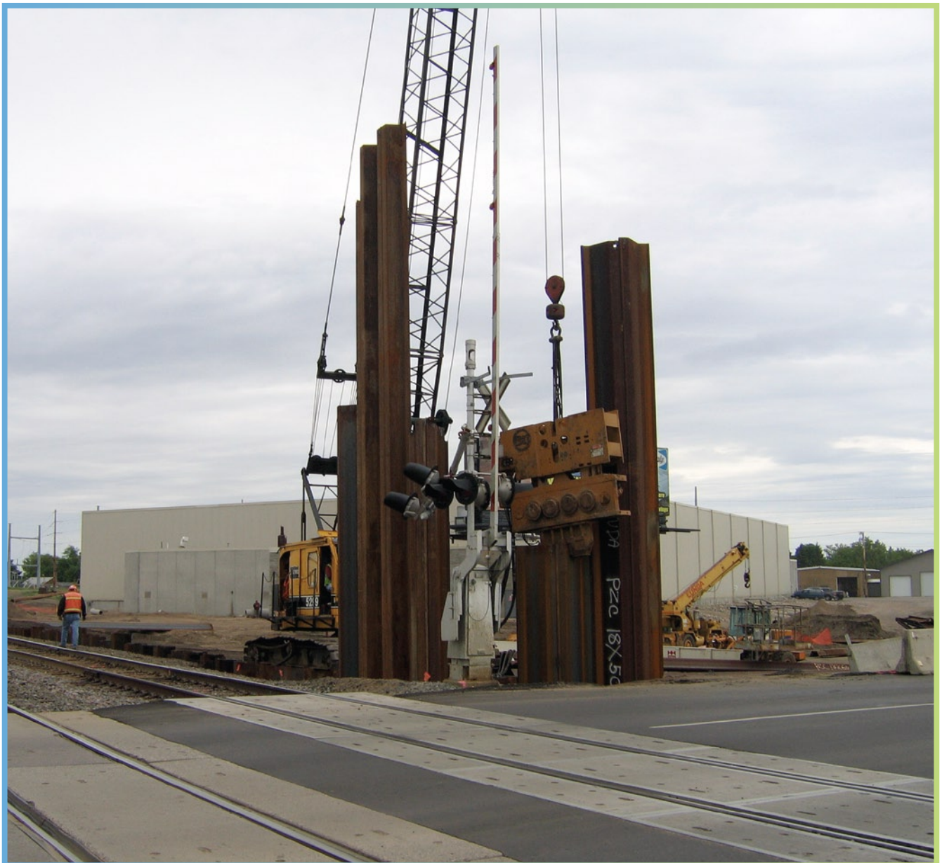
The Roosevelt Avenue Underpass sheet pile installation, located adjacent to the westbound rail, caused the most shift in the railroad track alignment. The monitoring system would send out an alarm if the shift exceeded .07 feet.
