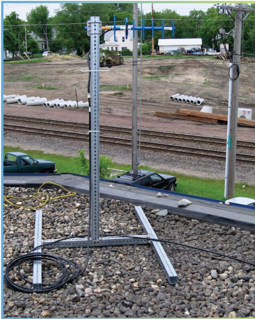
A yagi-antenna and a 900 MHz spread spectrum radio provided a clear communication link between the total station and the project computer located in a nearby project trailer.
