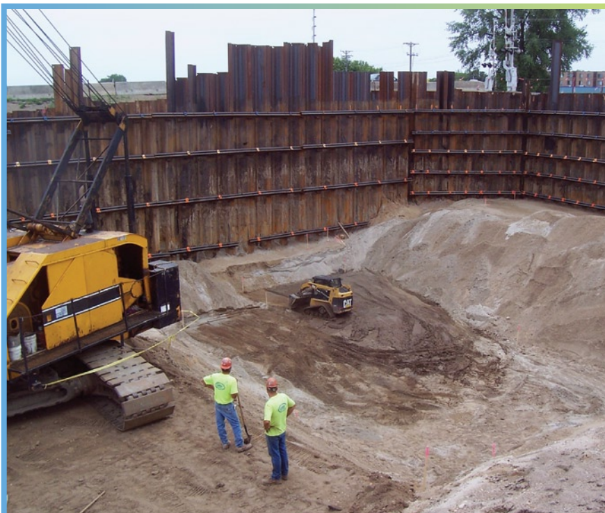
Mn/DOT surveyors and engineers relied on geodetic monitoring to track ground settlement during the excavation of the Roosevelt Avenue Underpass.
