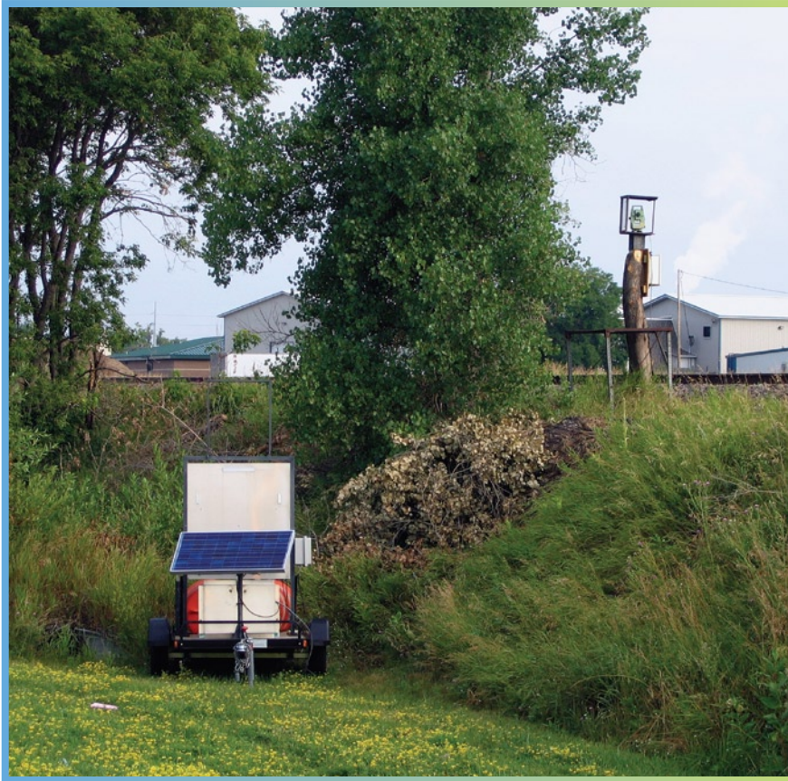
The mobile framework of the geodetic monitoring system allowed surveyors to set up even in areas with no power. This total station, located at Pelican River, is powered by a solar panel.
