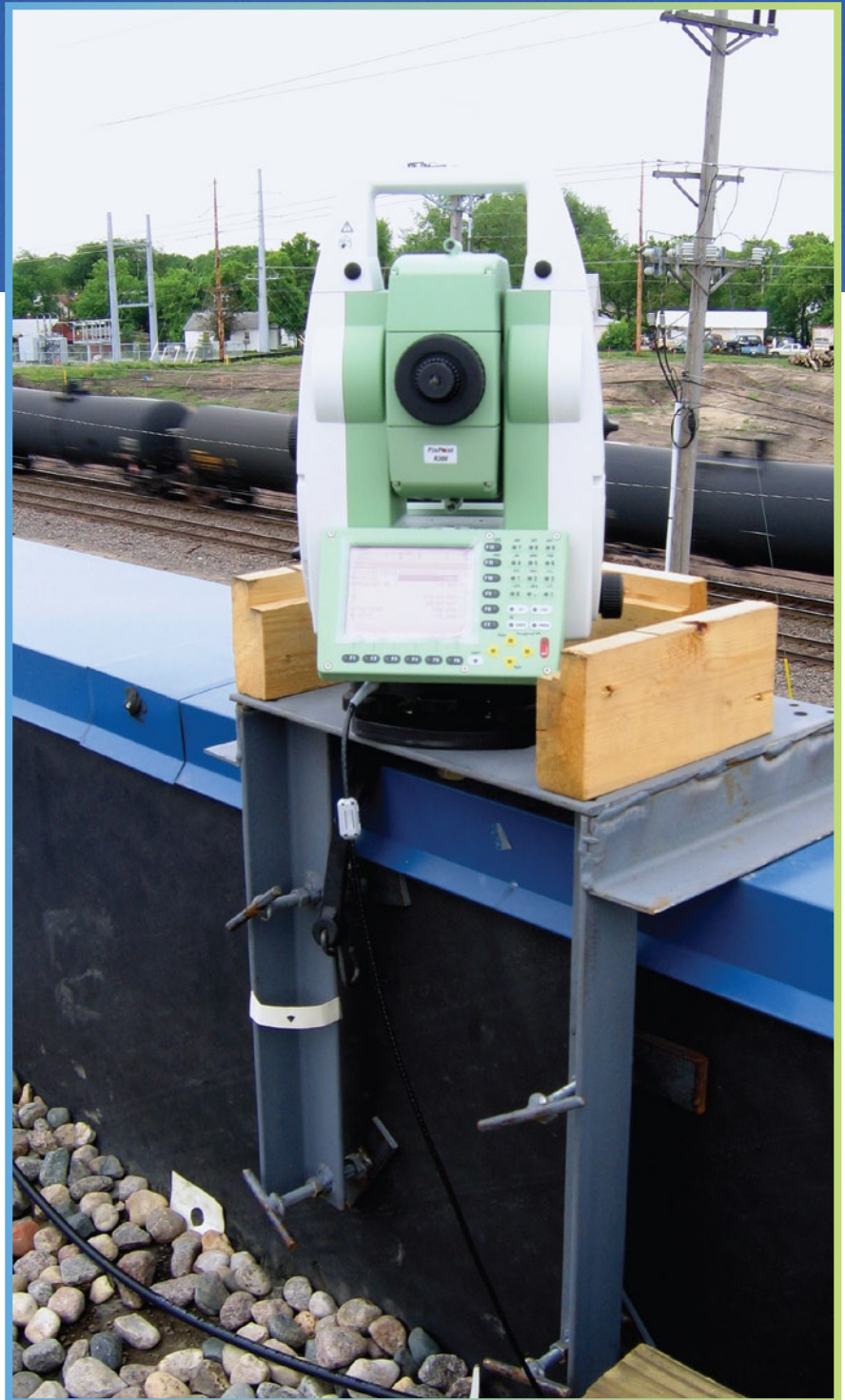
Surveyors relied on brackets that 'squeeze' the top of the wall to provide support for the total station and eliminate the need to drill holes in the building.
