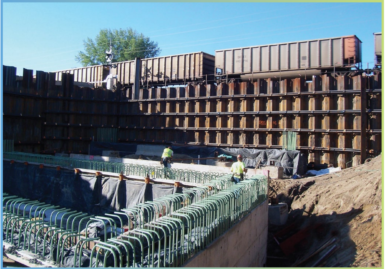
The Roosevelt Avenue Underpass infrastructure includes a storm water surge storage structure that is located beneath the new street level. The engineers called this the “boat section.”
