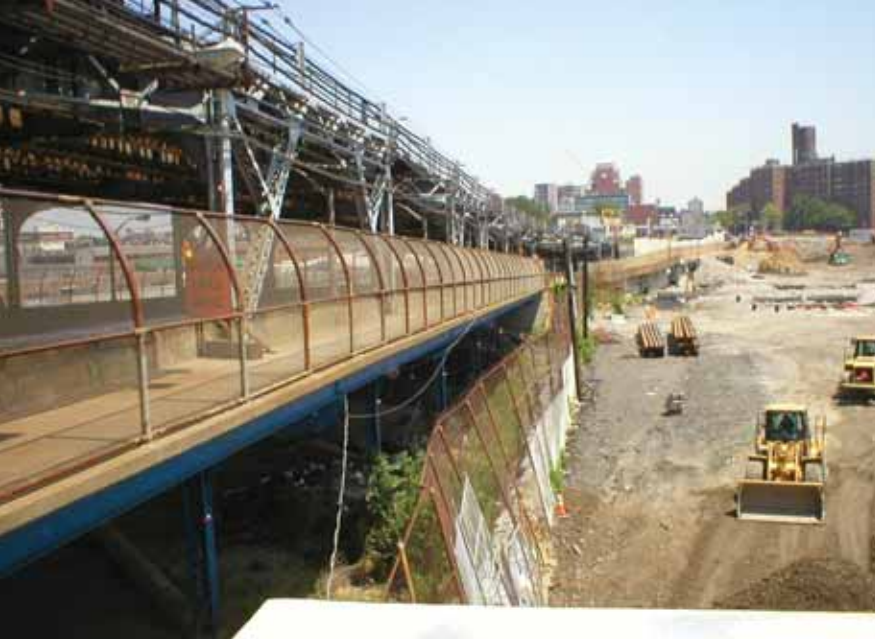
▲ Surveyors set up a monitoring network to track movement of subway tracks and a bridge during construction of a building
