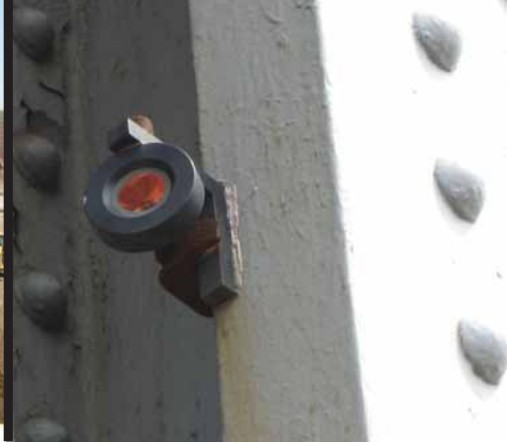
▲ Reflective prisms were installed with construction glue to the subway and bridge support structure
