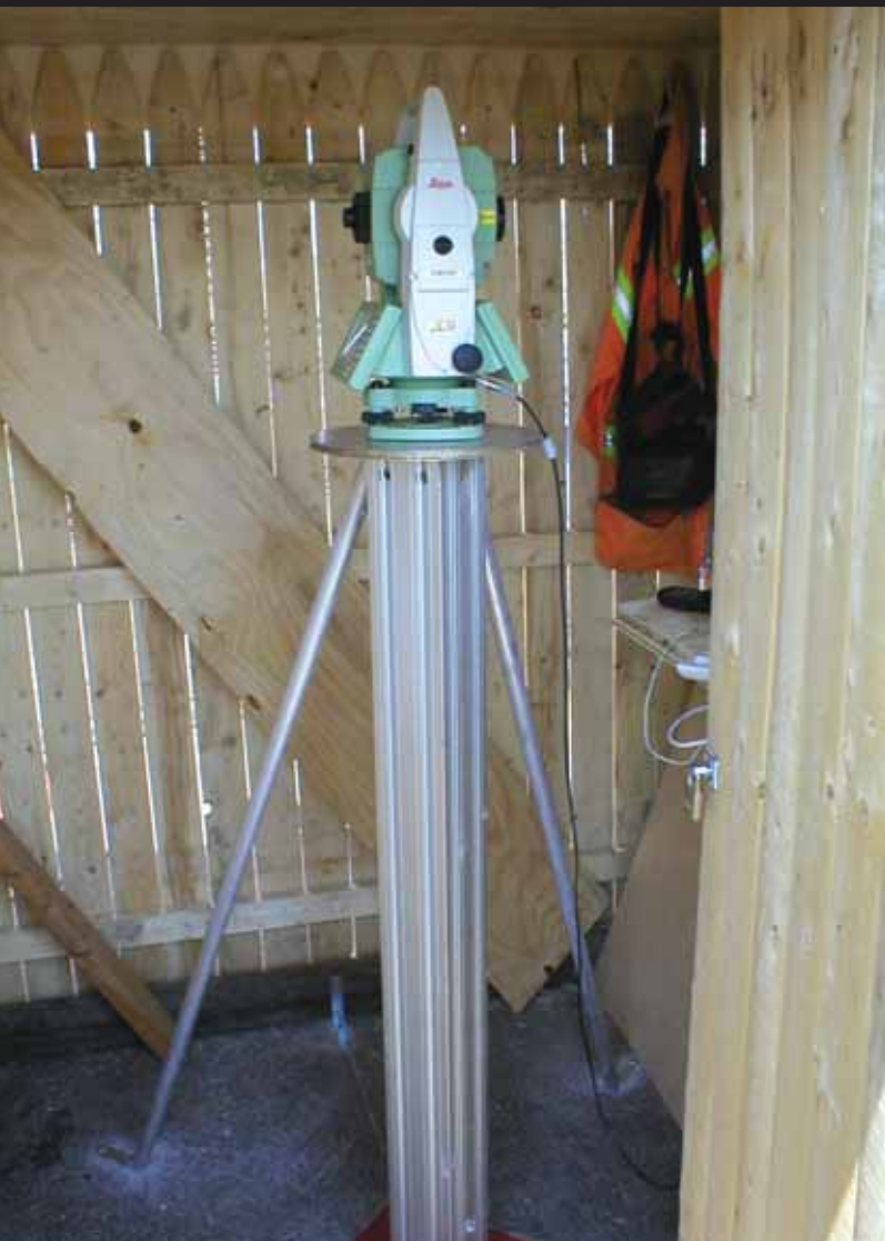
▲ A robotic total station was mounted on a custom-built pedestal permanently attached to a concrete bridge abutment and housed in a shed for protection
